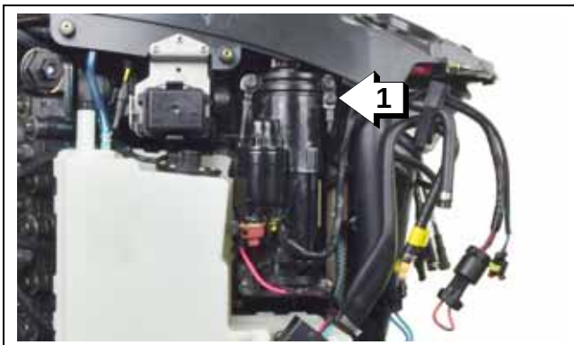
1. Main engine harness ground (Starboard) Located on upper starter bracket
