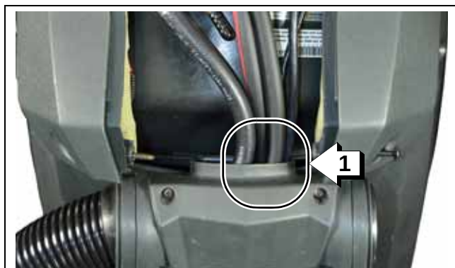
1. Cables NOT pinched
