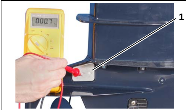
1. Meter lead to anode
